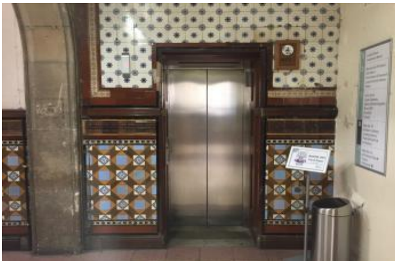
Ground Floor lift doors
