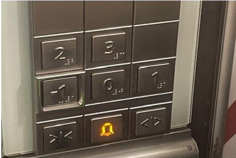
Interior lift buttons
