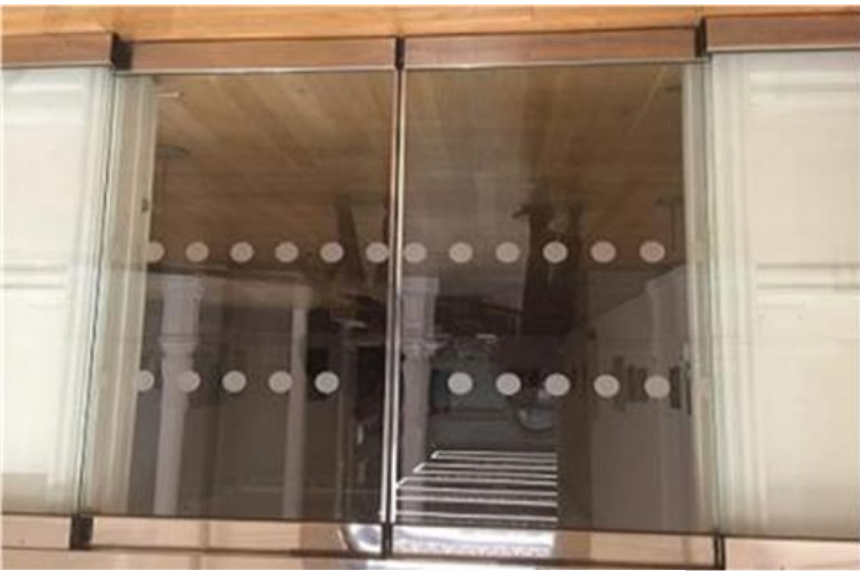
Contrast markings on some glass doors
